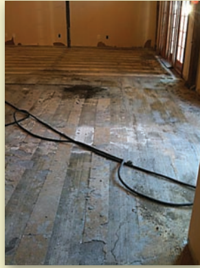
During the first grinding pass, the slab is ground in interlaced stripes to keep the depth even. Evidence of its deteriorated condition is plentiful.
