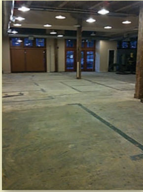
The slab in the 103-year-old building bore evidence of many past lives. It was of different colors, had cracks and heaves, and was covered in layers of mastic.
