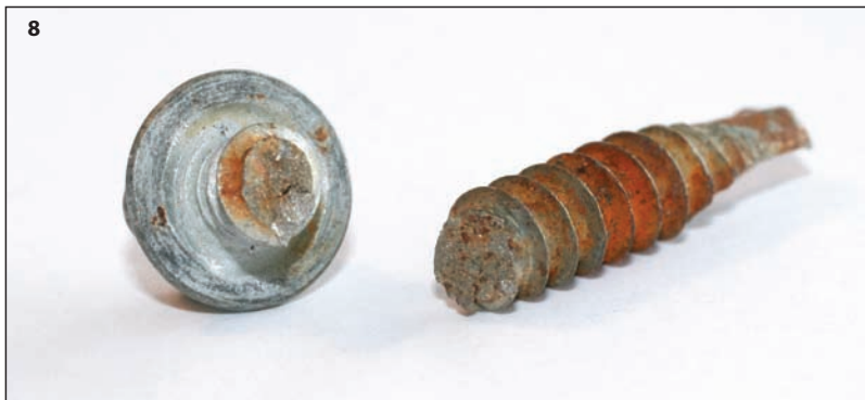
Photo Courtesy of Elco Construction Products, an Acument Global Technologies company
